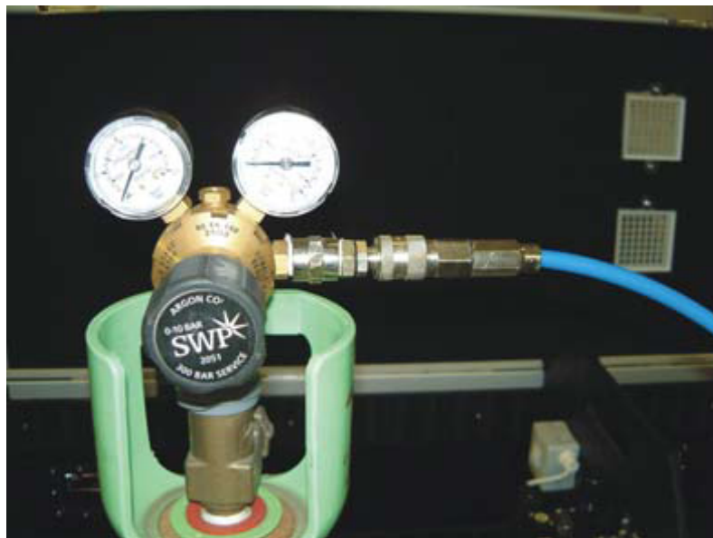
This shows the connection of the (blue) pneumatics hose to the regulator and the regulator to the bottle of compressed inert gas such as nitrogen, carbon dioxide or compressed air.
